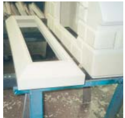
Figure 9. Preparing to glue the base to the main body with urethane glue
