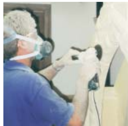
Figure 11. Grinding the stone effect into the faces using a 4-in. grinder. (This goes fast, but it's messy!) Be careful not to hit the mortar.
