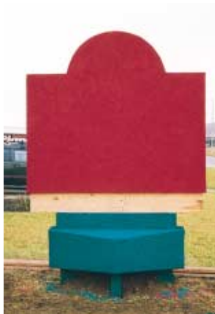
Figure 13. After the finish coat dries, the structure is ready for the trim and sign panels.
