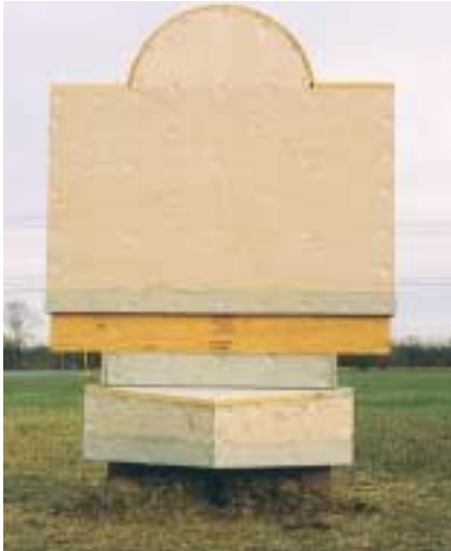
Figure 7. After the insulation board is installed, the sign is ready for stucco.
