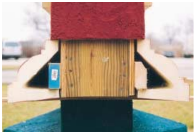
Figure 14. The architectural moulding at the bottom of the main panel was installed with stainless steel screws.
