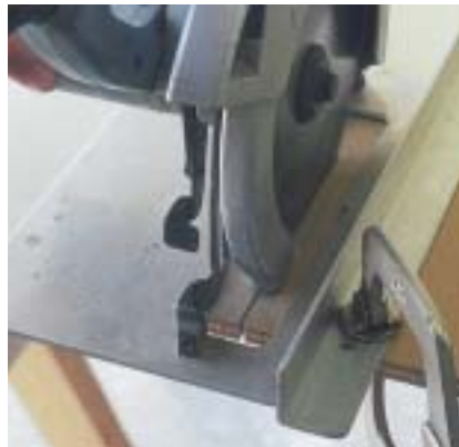
Figure 2. The blade of the circular saw is adjusted so that about 1/8 of an inch runs below the MDO. Since the panel is on wooden sawhorses, the only damage is a small groove in the support. A sharp blade makes quick work of slicing off our panel from a 4-by-8-ft. sheet.
