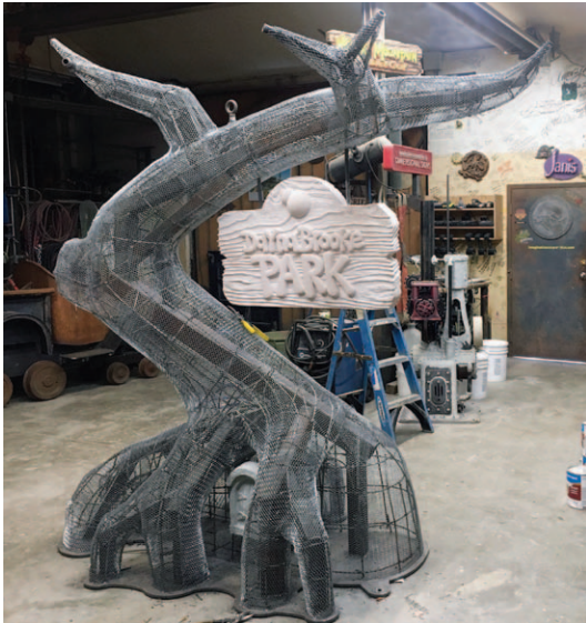
The tree is now wired and ready for concrete. The edges of the sign were textured with a die grinder to extend the woodgrain seamlessly from both sides. This small detail adds a lot of believability.
