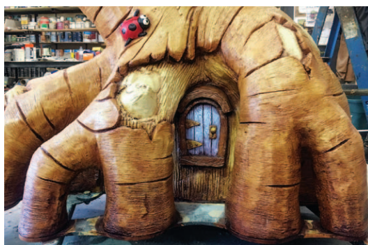
The many roots of the tree add interest to the feature—and most of the complexity to the project. Welding the armature, tying on the lath, applying the concrete and sculpting it, along with the painting are all much more difficult and time consuming in the back and upside-down areas. The fairy door was done using sculpting epoxy for extra detail.
